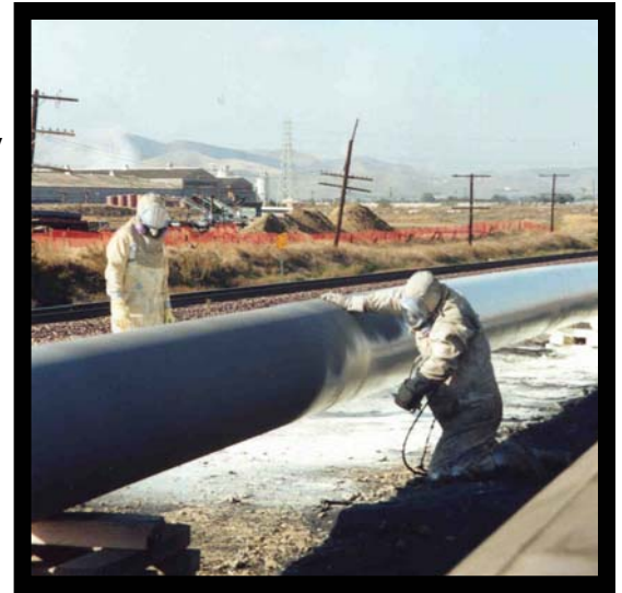
Field application of EF-RBU over steel pipe Blasted to SSPC-SP10 "Near White" Blast
